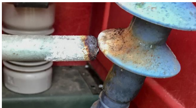
Degraded termination is obvious
