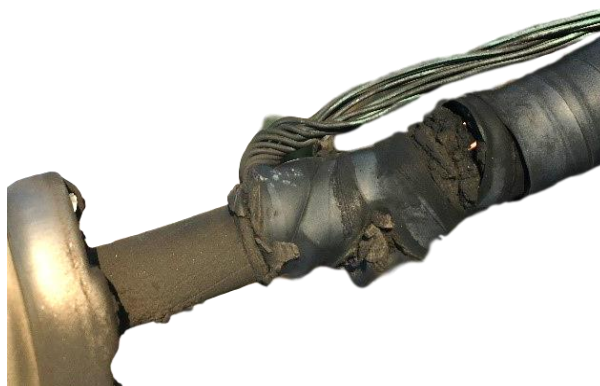
Degraded termination causing PD
