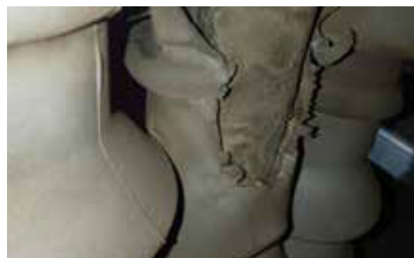
Damage to the polymeric insulation of the 33kV cable termination due PD activity.
