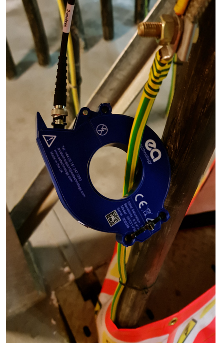
Figure 4: HFCT on earth braid of HV cable
